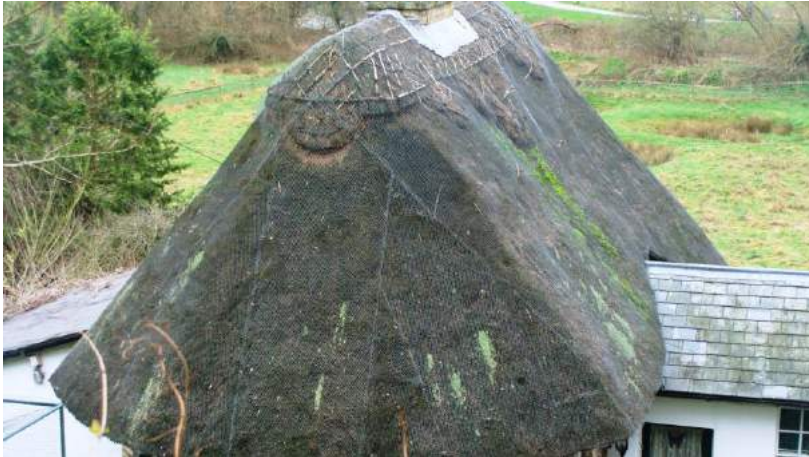
Picture 99. The Vineyard - thatched ridge appears in need of repair which may be eligible for EHDC grant assistance.
