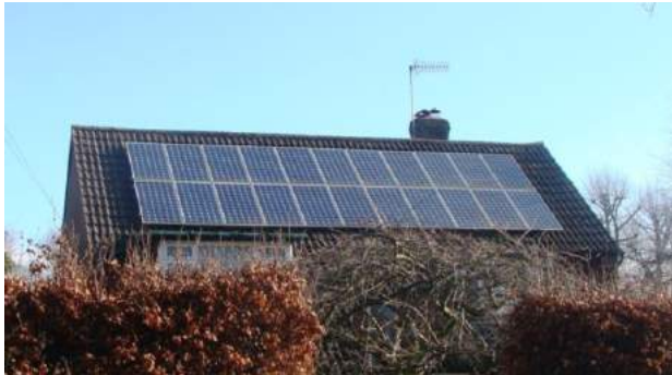
Picture 132. Another example of solar panel on a modern building in the conservation area.
