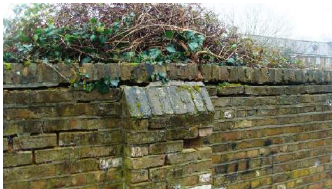
Picture 96. Wall at Pilleway Pitteway Walk in need of repair.
