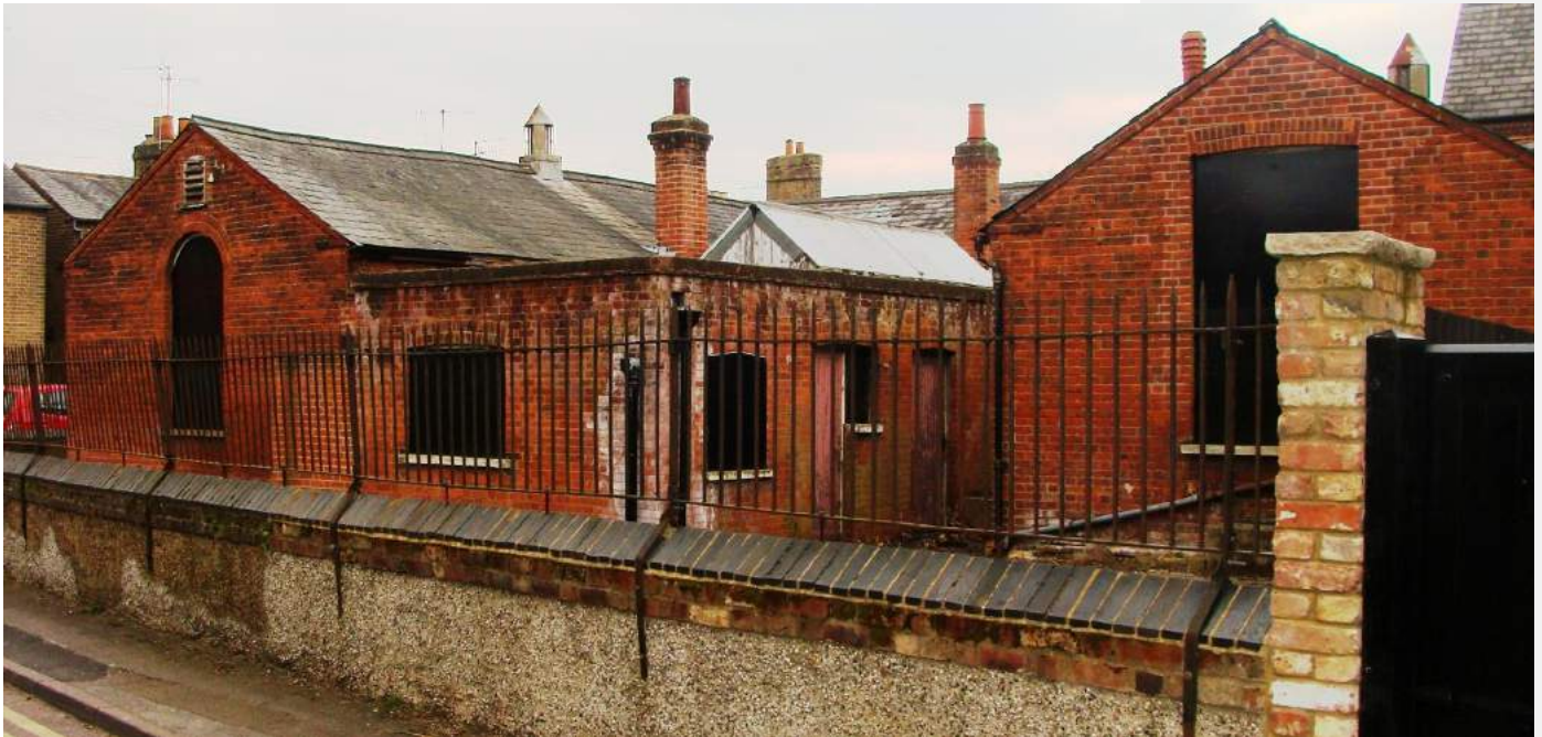
Picture 44. Part of a larger site at Dimsdale Street that is cause of concern and in need of further investigation before concluding its future.
