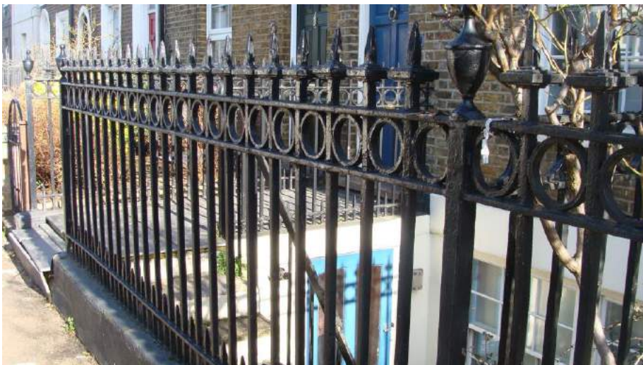
Picture 173. High quality railings to front of Nos. 14 -16 Villiers Street. Note basement accommodation below ground level.
