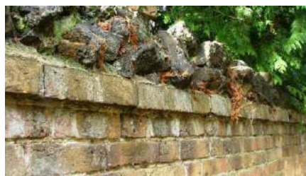
Pictures 140-141. Good quality bollard probably dating from the 19th century and brick wall capped with industrial clinker waste defining public footpath 82. An important and well used component of the urban scene.
